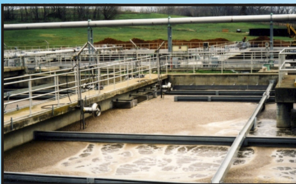
Effluent Treatment Plant
